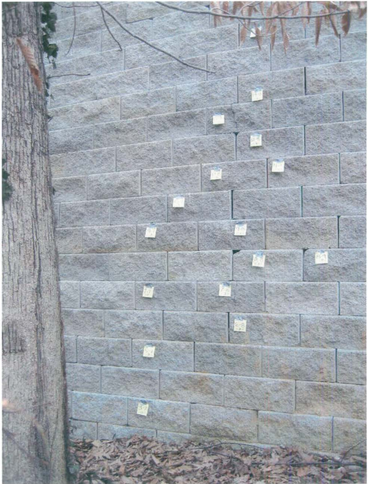
Examples of Cracks Developing Systemmatically in groups of mesa blocks (c 2/13/05)
