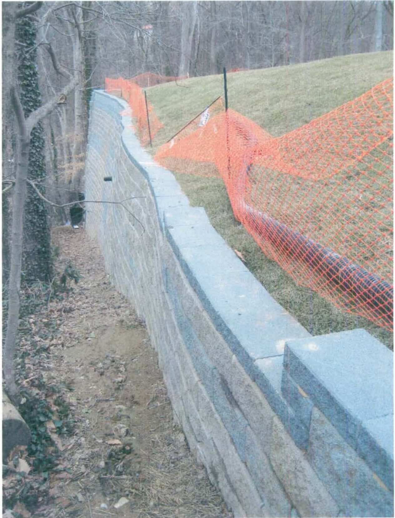
View of bulges and undulations in wall.
