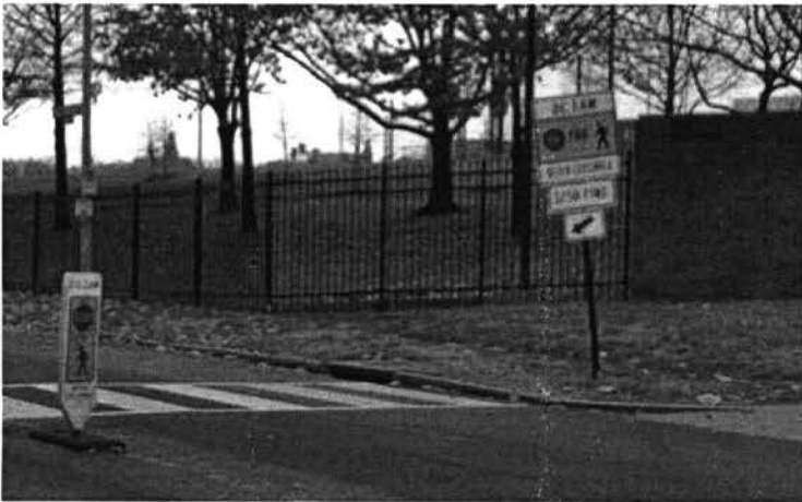
Figure 9: Missing Curb Ramp along West Virginia Avenue just south of Gallaudet Campus gate
