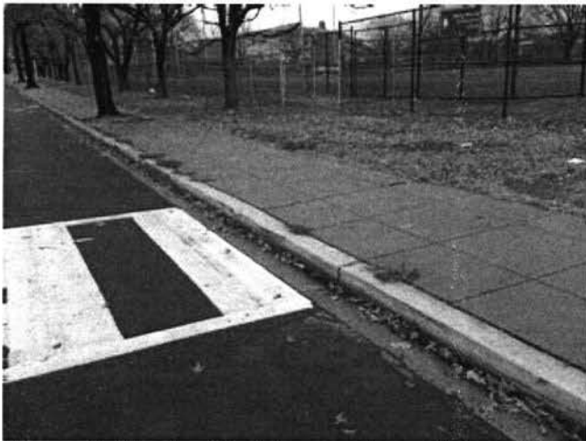
Figure 8: Missing Curb Ramp along 6 th Street just north of Gallaudet Campus gate
