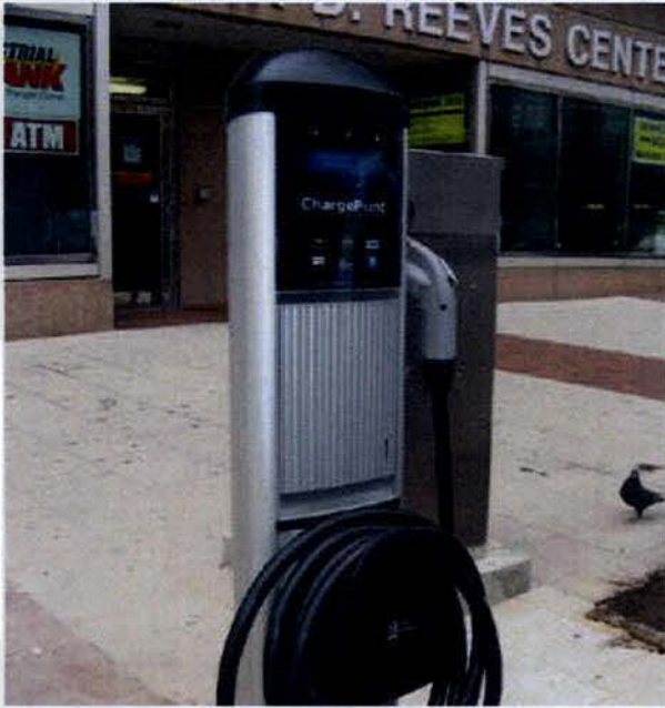
Figure 2.37: Electric car charging station near 14th and U, NW.
