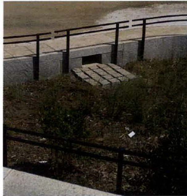
Figure 2.32: Biofiltration system near the Navy Yard.
