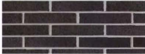
BRICK 2 - AT BUILDING BASE ON CUSHING PLACE ALLEY
