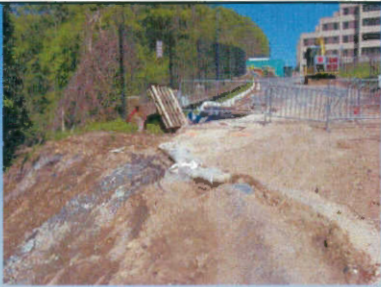
The collapsed slope in April 2010. Georgetown University has built a retaining wall below the road.
