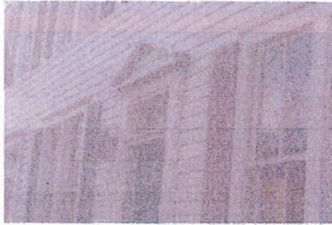
Aluminum siding, running full length of three properties (does not meet historic district code)
