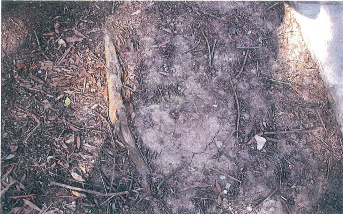
Photograph 5 – Damage of exposed root associated with Tree 2. Note orange-colored fungus on root which may signify decay.
