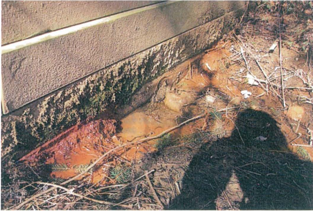
Photograph 3: Existing groundwater seep/ spring originating from existing retaining wall on Canal View community property.
