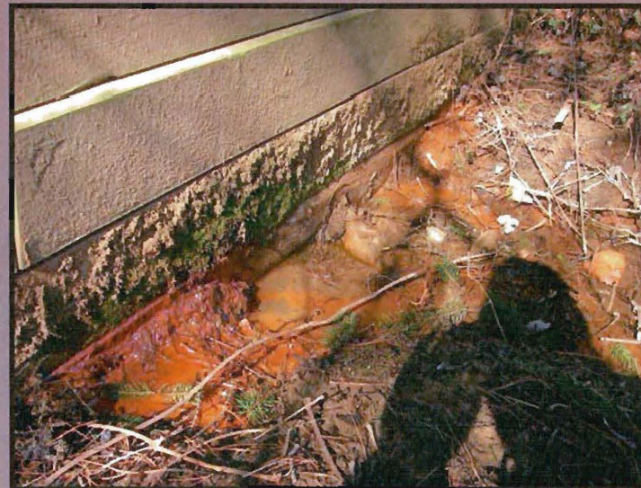
Seepage under Canal View ret. wall
