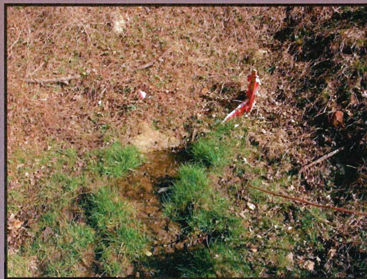
Groundwater seep near basketball court
