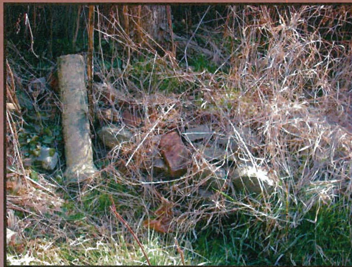
Groundwater seep near Ligan Way
