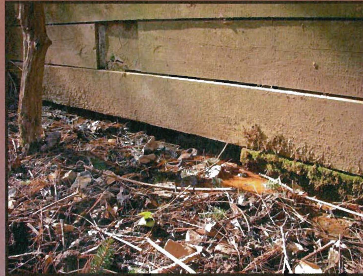
Seepage under Canal view ret. wall
