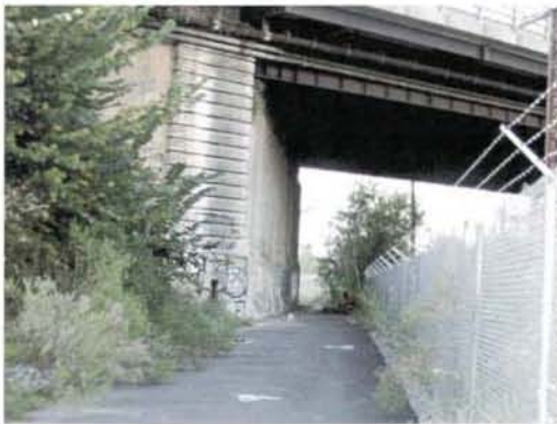
Existing Change of Grade at New York Avenue
