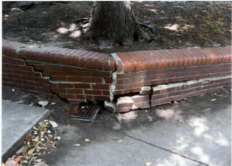
Figure 2 Damaged brick retaining wall
