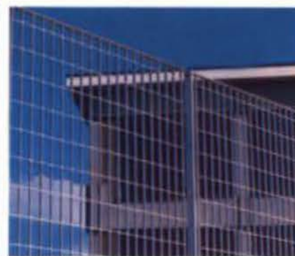
STEEL FENCE at EXISTING PARKING AREA
