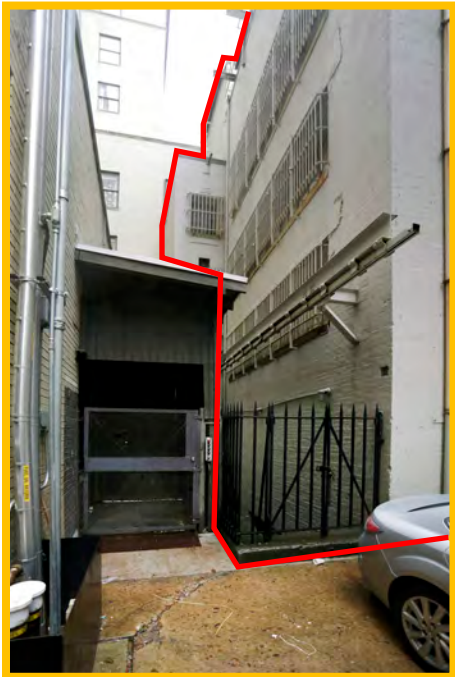
ENLARGED VIEW OF EXISTING NON-COMPLIANT REAR YARD
