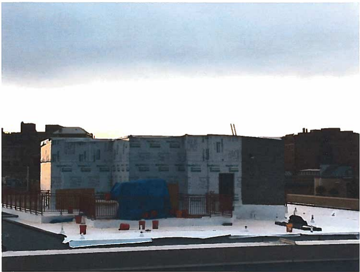
This photo was taken on 2/7/16 from my roofdeck and shows the completed cap on top of the penthouse and the complete blockage of my view of the Cathedral.
