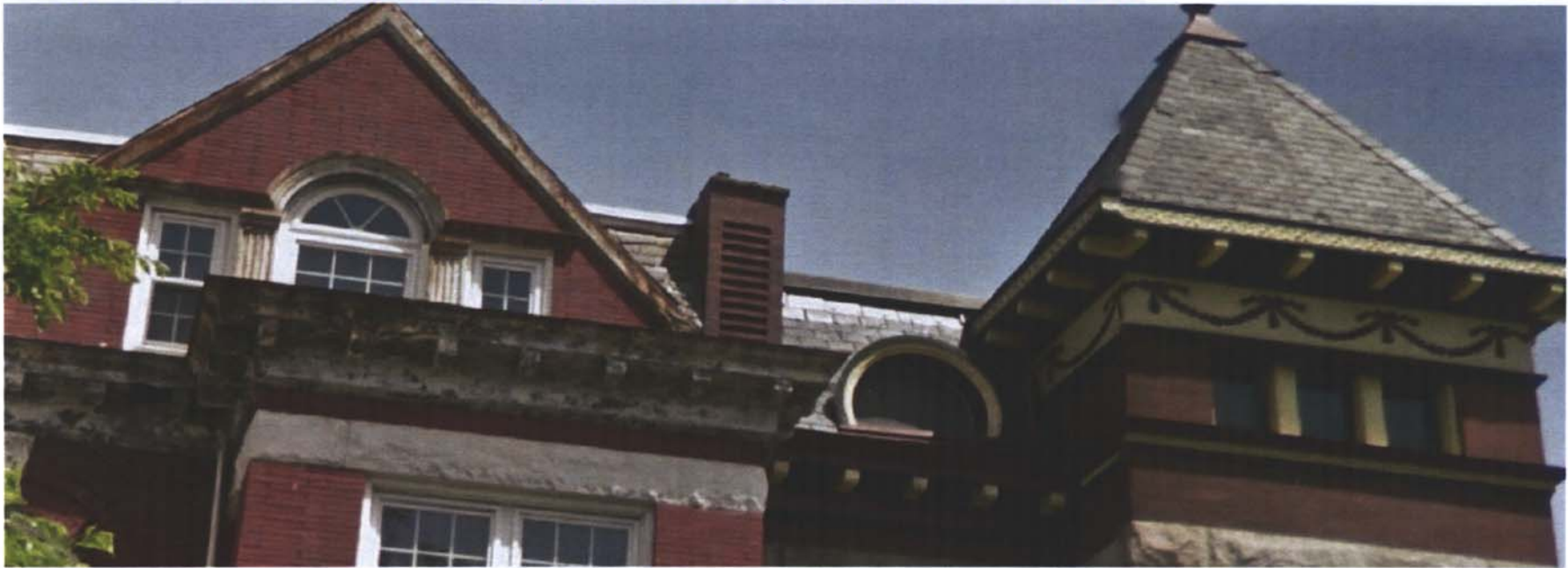
EXCEPTIONAL CONDITION: LEVEL OF DISREPAIR/STRUCTURAL ISSUES/PROLONGED BLIGHTED STATE
