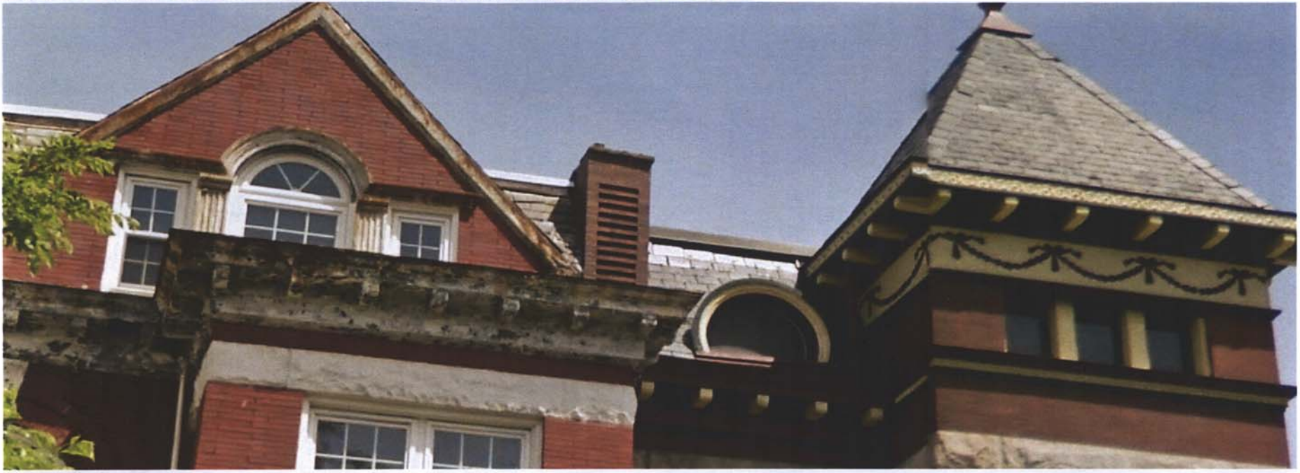
LEVEL OF DISREPAIR & STRUCTURAL ISSUES CREATES EXCEPTIONAL CONDITION
