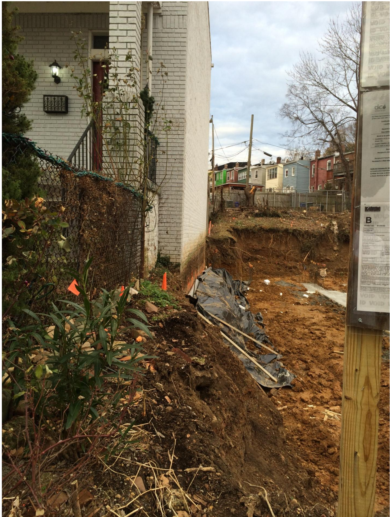
December 21, 2013, 9:12am. Before property damage public space. Front view.
