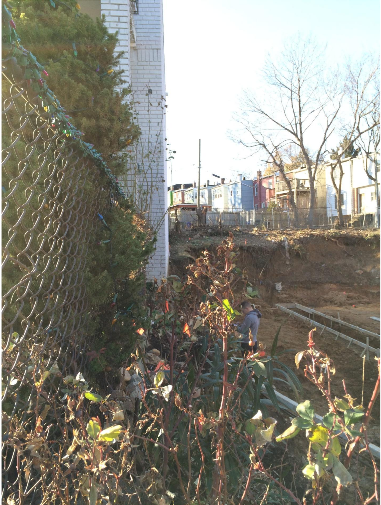
December 16, 2013, 3:16pm. Our Structural Engineer & Front view public space before damage.
