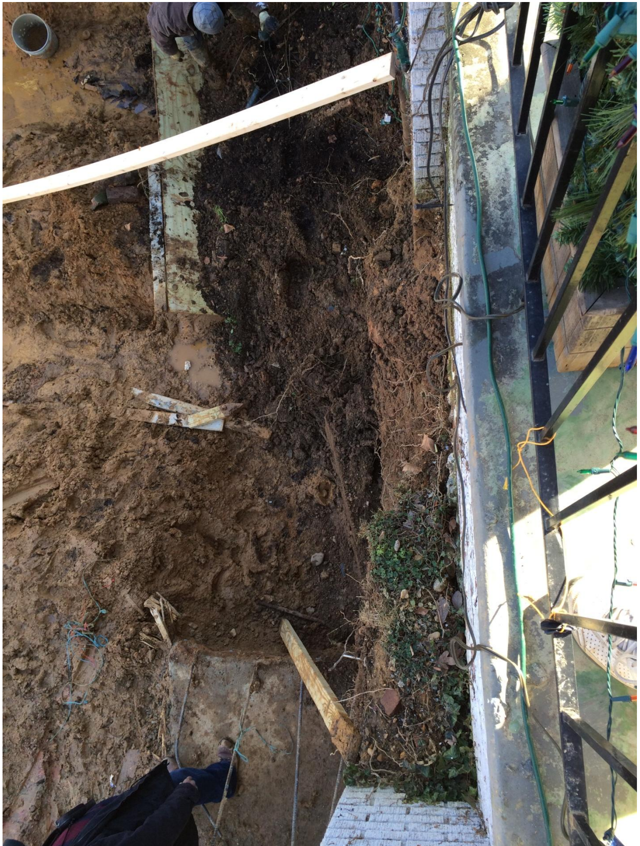
January 13, 2014, 11:11am. Top view 2110 3rd St NE property/public space missing.
