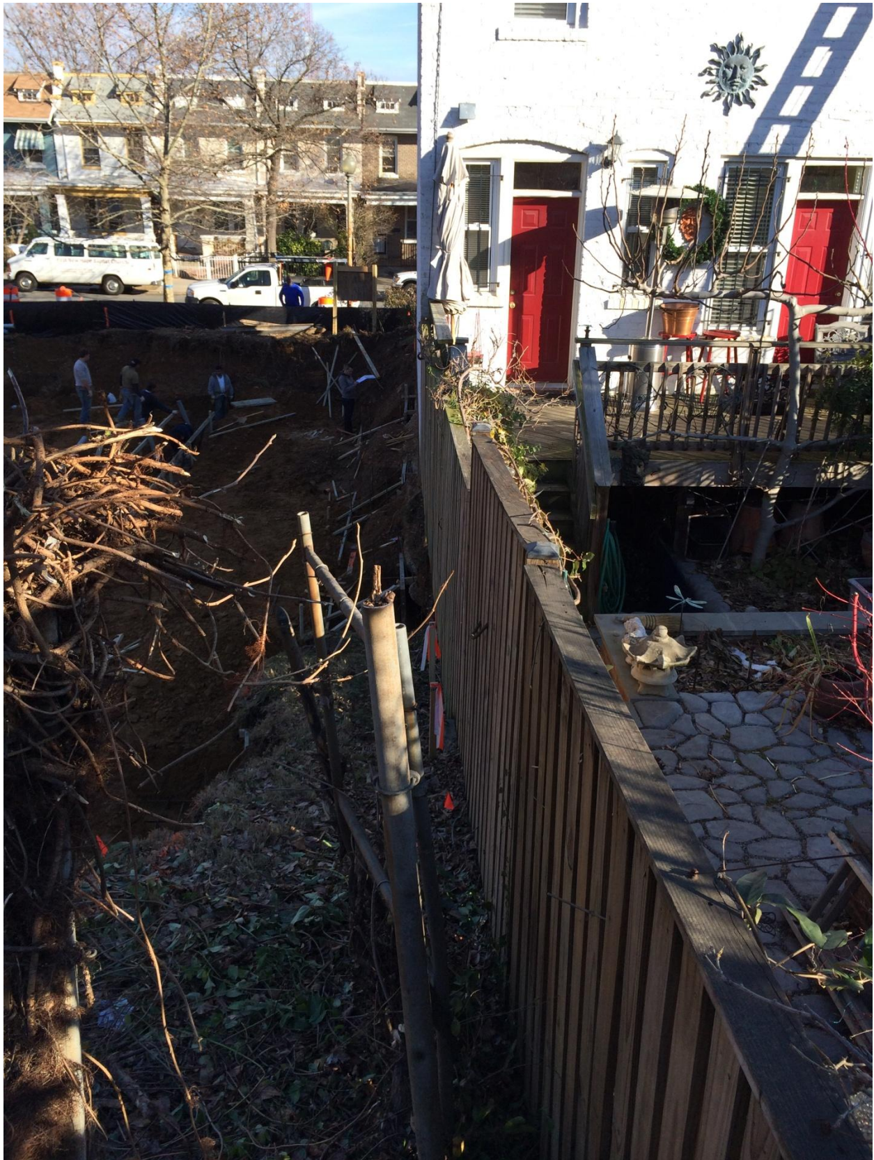
December 19, 2013, 3:14pm. Before damage and encroachment into our property.
