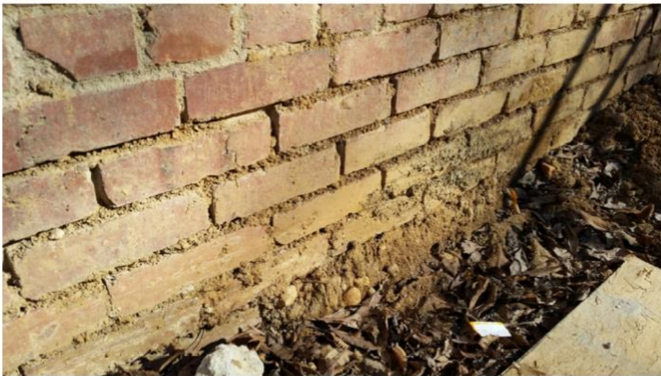
Photo #4 – Deteriorated Mortar in wall between 1828 and 1830.
