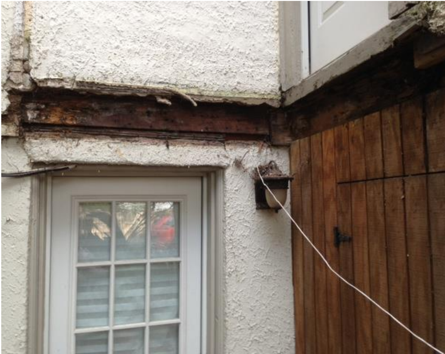
Water damage from old deck over our shed and basement door (has since been repaired.)
