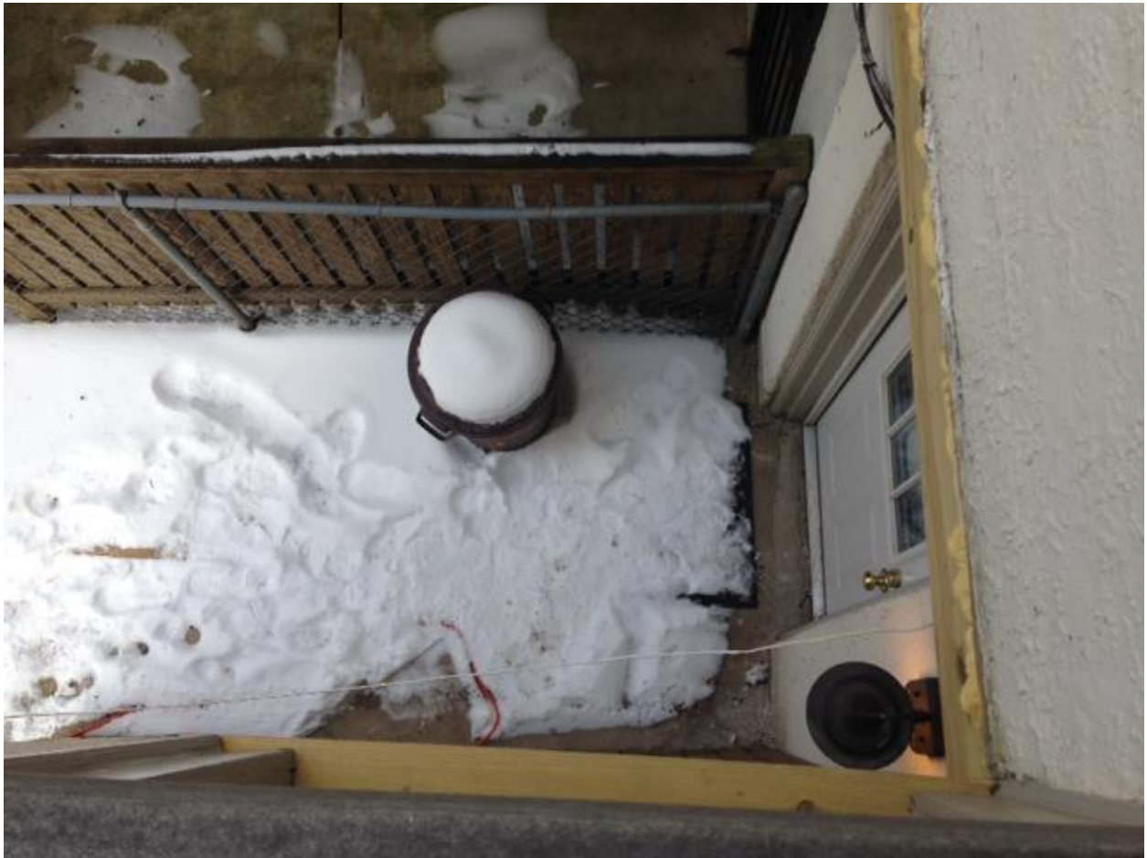
View out of kitchen door down to ground one story below, showing current hazardous condition in absence of deck (which worries us as we have two small children.)
