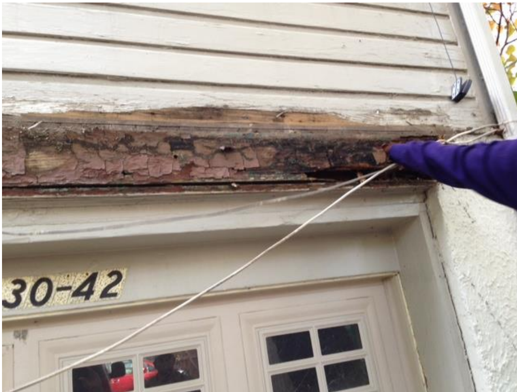
Water damage from old deck caused terrible rot, and has since been repaired.
