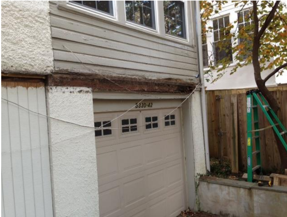
View of rotten wood over our garage, which was behind the old deck and has since been repaired.
