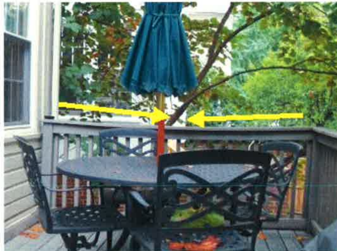
sagging rear deck.
