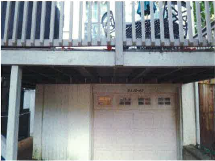
Sagging rear deck.
