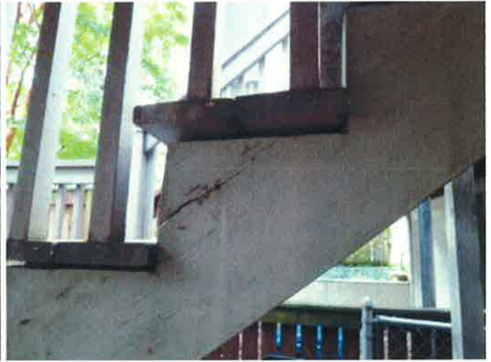
Deteriorated stairs at rear wall.
