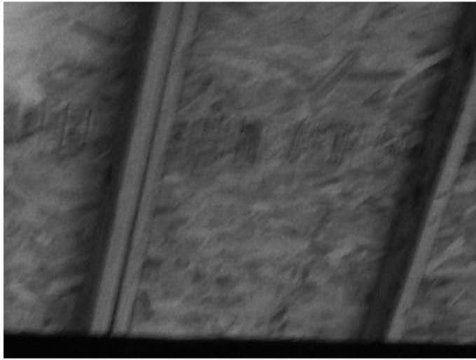
Fig. 7: Roof Joists Spaced more than 24" o.c.
