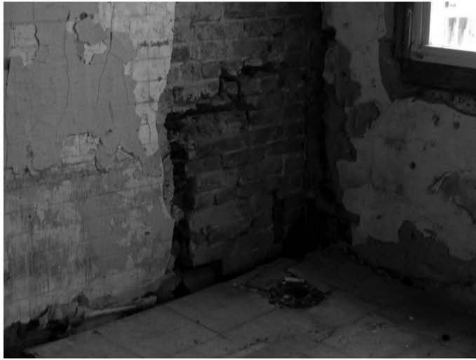
Fig. 1: Deteriorated Rear Wall
