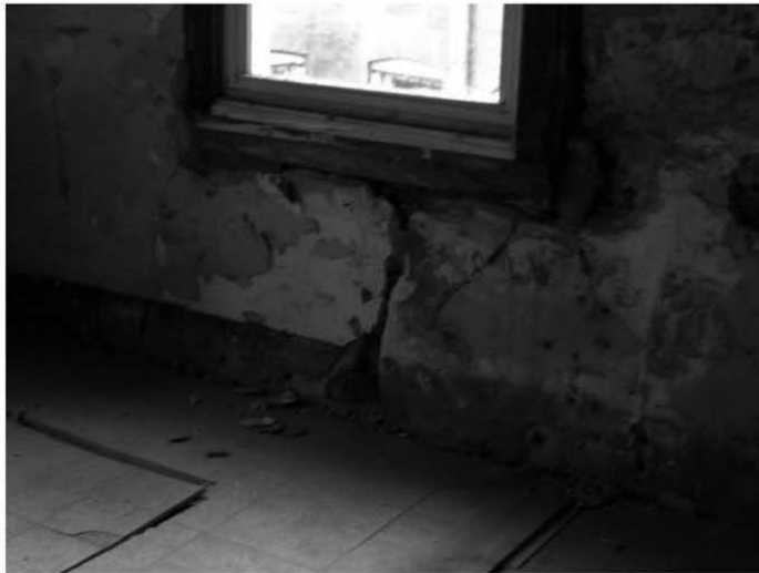
Fig. 8: Settlement Crack at Right Side Wall @ Rear
