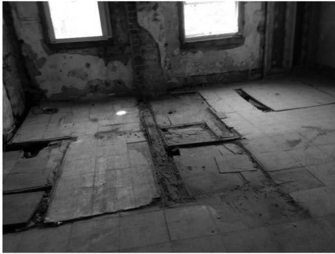
Fig. 5: Rear of the House Deteriorated
