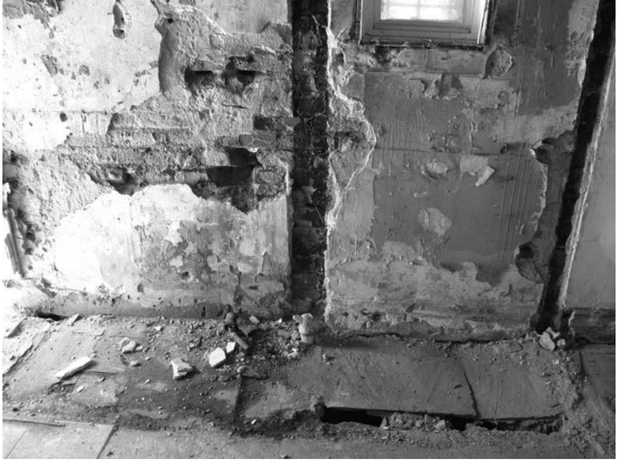
Settlement and deteriorated state of Western bearing wall
