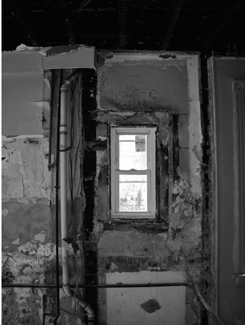
Deteriorated state of the building carefully hidden by the previous owner were uncovered. Structural damage over time requiring unforeseen and costly structural repairs.
