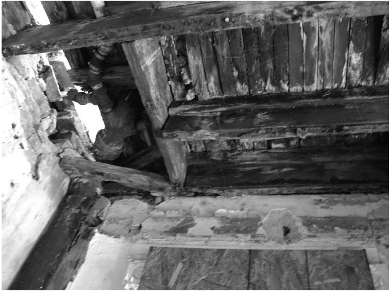
water damage and rotten wood joists creating unsafe conditions.
