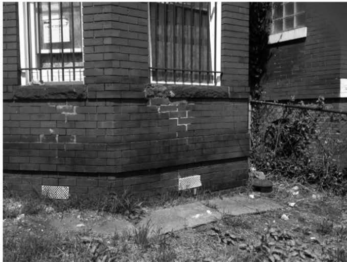
Fig. 2: Settlement Cracks in Front Wall
