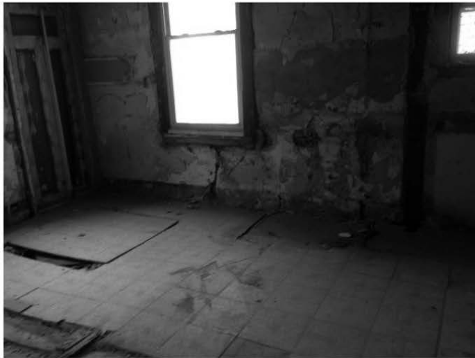
Fig. 6: Mortar Deterioration @ Right Side Wall @ Rear
