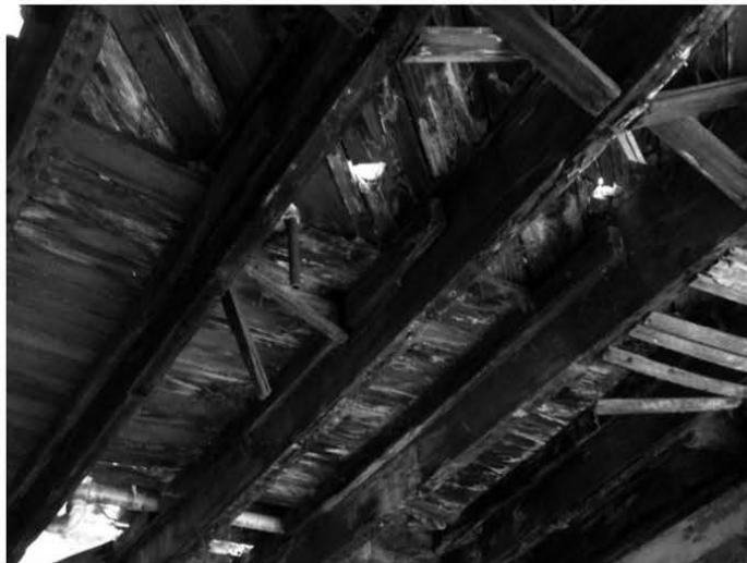
Fig. 10: Floor Joists damaged due to water @ Second Floor
