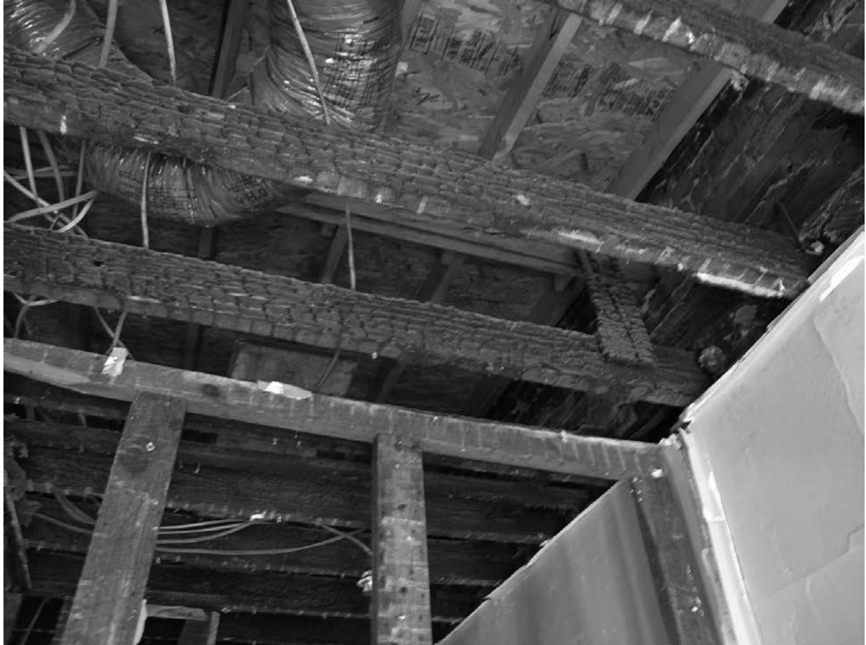
Fire damage and improperly installed electrical wiring and roof structure, testament to the property's history of unsafe maintenance.
