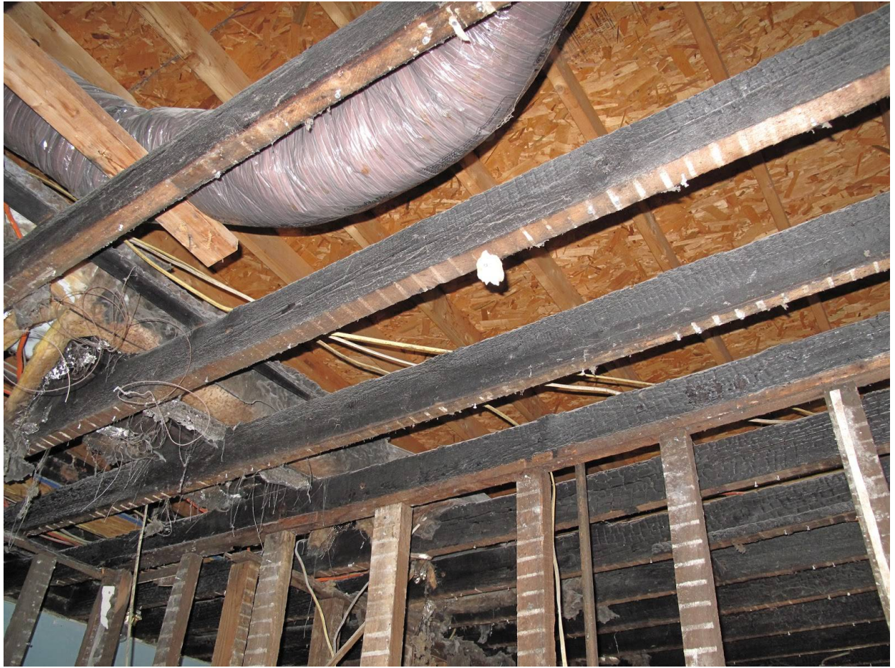
Extensive fire damage caused by two separate fires.
