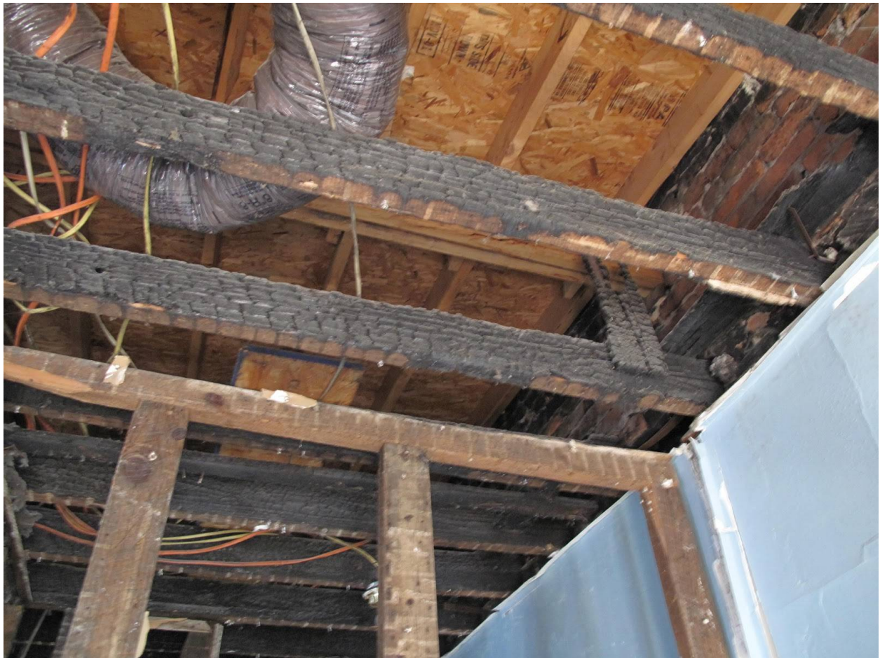
Joists showing extensive fire damage. Improperly installed electrical writing a testament to the property's history of unsafe maintenance.
