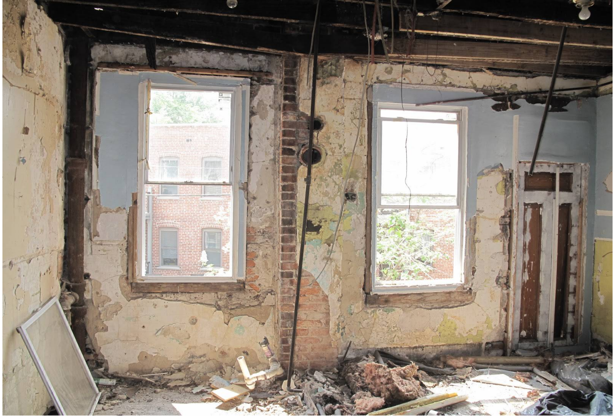
Broken roof joists and dilapidated condition of bearing walls.
