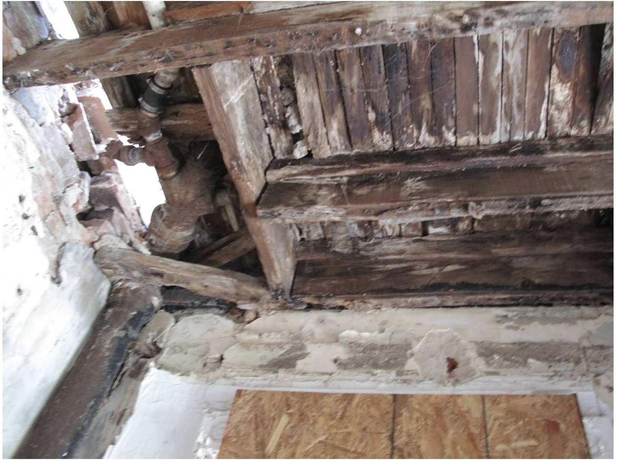
Improperly installed and rotten wood joists creating unsafe conditions.
