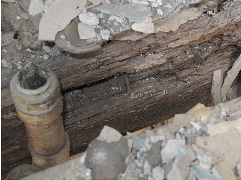
Joists showing moisture damage.
