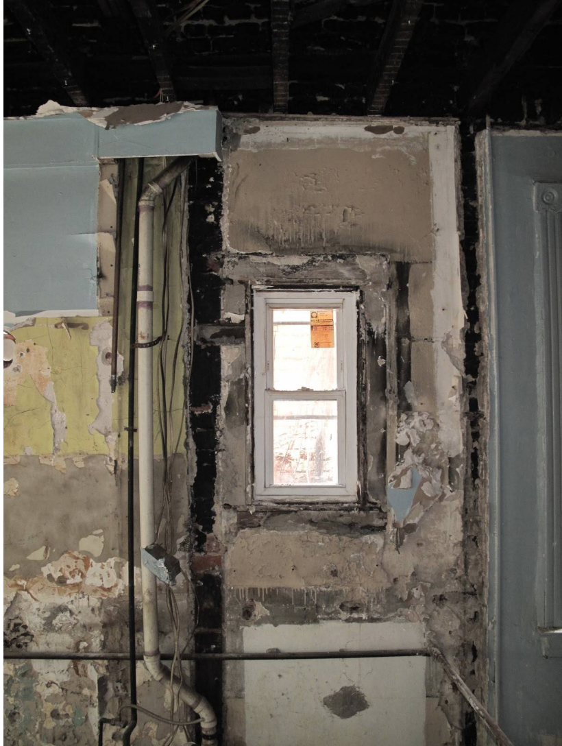
Neglect and non-existing maintenance of the building causing structural damage over time requiring unforeseen costly structural repairs.
