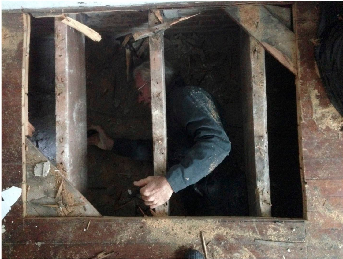
Home inspector George Pettie inspects floor joists and crawl space.. He finds numerous improperly repaired and damaged joists. Repair of the joist, missing insulation and structural reinforcements require full replacement of the floor and subfloor.
