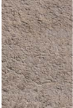
Plaster at niche walls & upstairs walls
