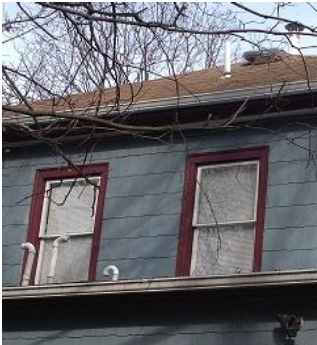
South side – four vents
