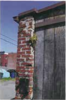
South Plywood Wall – Inside and outside view: open to rodents and in need of repair
