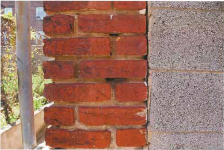
Gap around loading dock cinderblock – cinderblocks are leaning into the alley.
