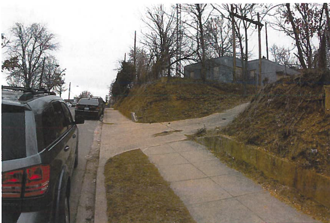
ON 4TH STREET SE, Southwest corner of the property adjacent to existing drive/ curb cut looking North. Showing existing chain link fence, side walk, 18 inch retaining wall, steep grade change, erosion issues on inadequate retaining wall. Note the change in elevation from the sidewalk to what appears to be the flat portion is 13 feet, occurring in about 8 foot distance.
