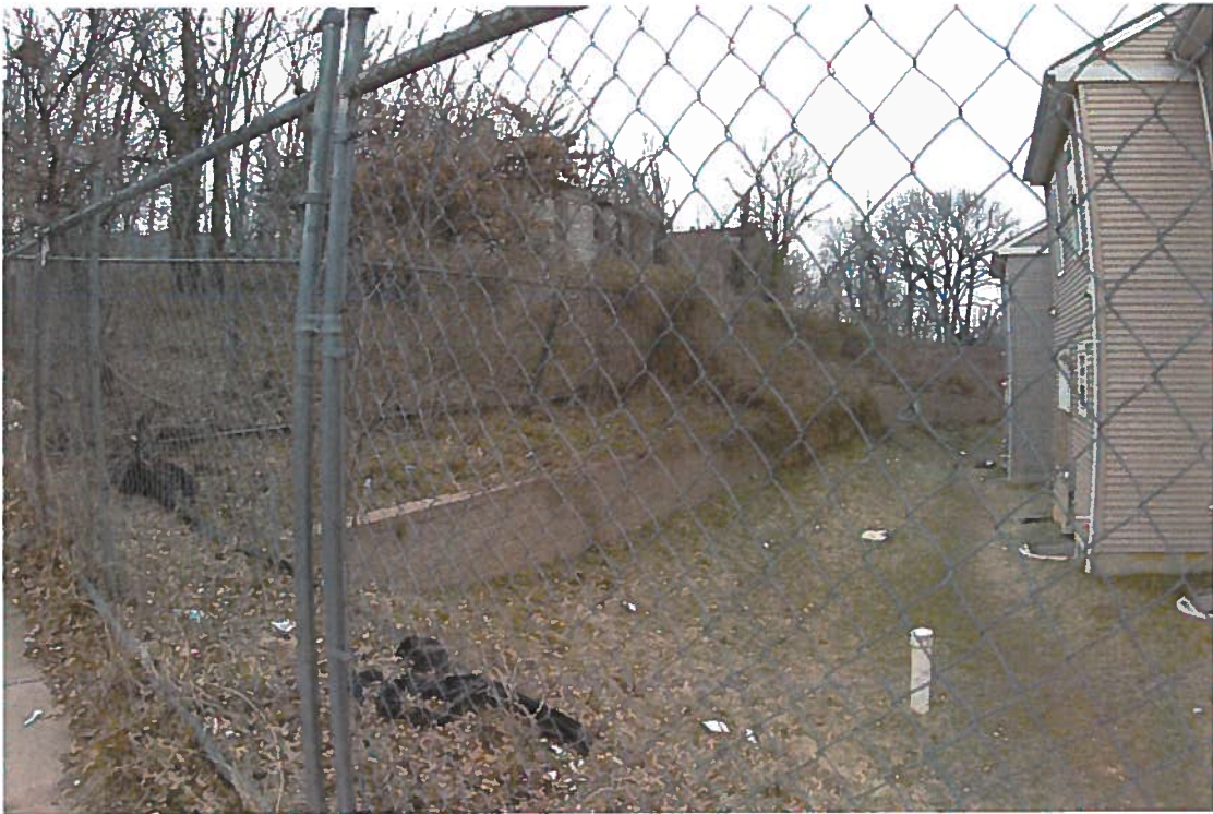
ON 4TH STREET SE, Southwest corner of the property looking Northeast. Showing South property line, back yard of adjacent to residential, retaining wall and existing failing chain link
