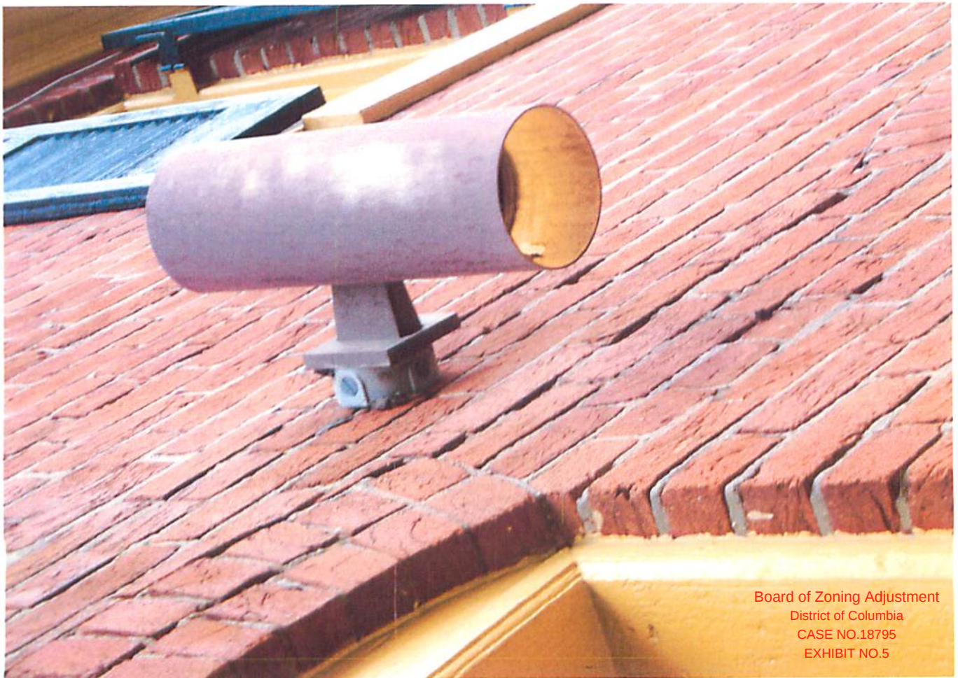
EXISTING LIGHT FIXTURE
