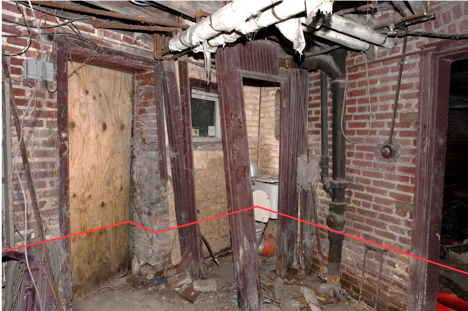
WATERLINE, BELOW WHICH THERE WAS STANDING WATER
