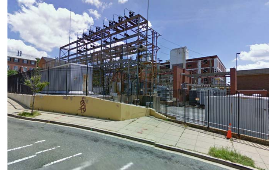
PEPCO Facility Along Champlain St
