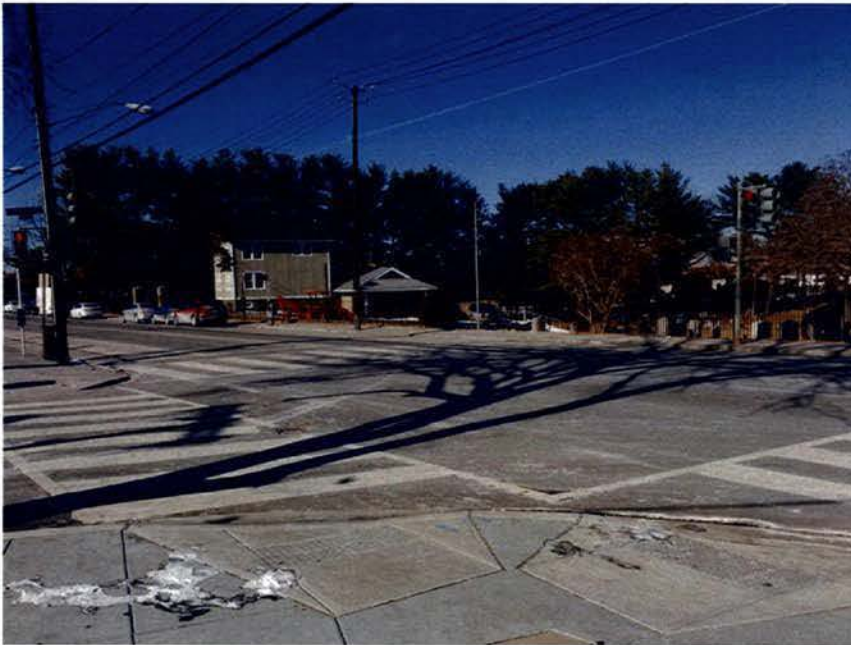
Figure 12: Pavement Conditions: Alabama Avenue and Congress Street (looking northwest)
