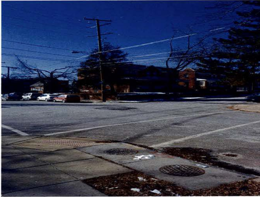
Figure 9: Pavement Conditions - 13 th Street and Savannah Street (looking southwest)
