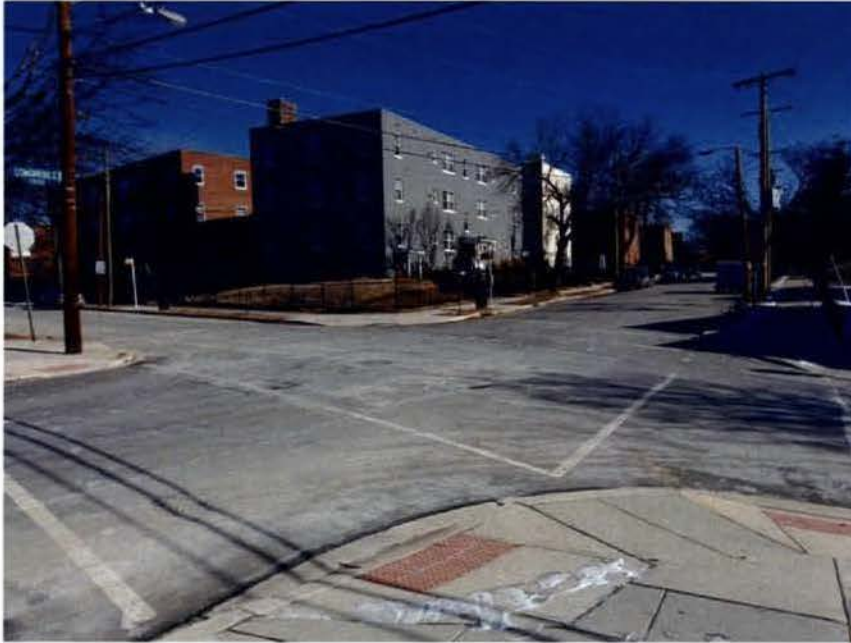
Figure 10: Pavement Conditions - 13 th Street and Congress Street (looking northeast)
