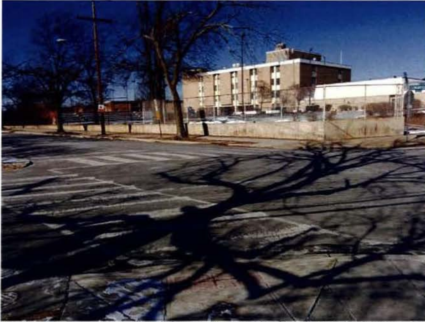
Figure 11: Pavement Conditions: Savannah Street and Congress Street (looking northwest)
