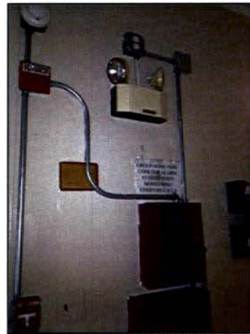
EXPOSED COMMERCIAL FIRE EQUIPMENT
