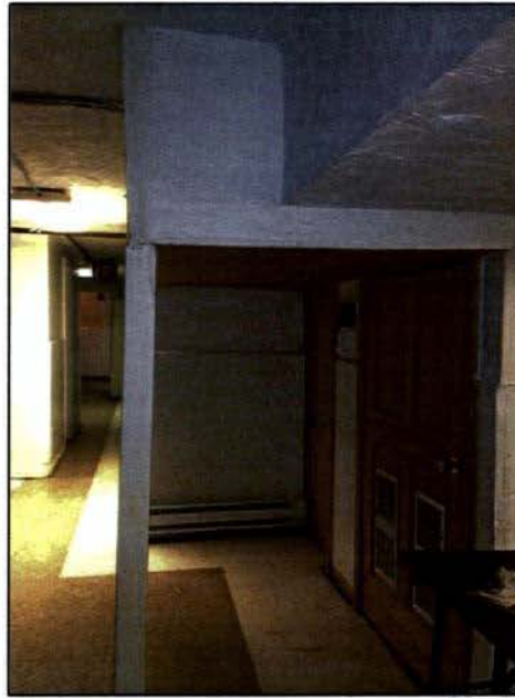
AWKWARD CEILING IN BASEMENT
