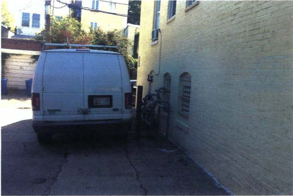
EXHIBIT ② UNPROTECTED GAS LINE
