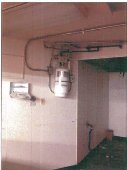
EXHAUST HOOD AND GAS LINE
