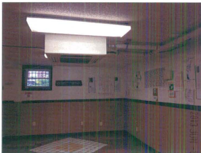
COMMERCIAL HVAC SYSTEM
