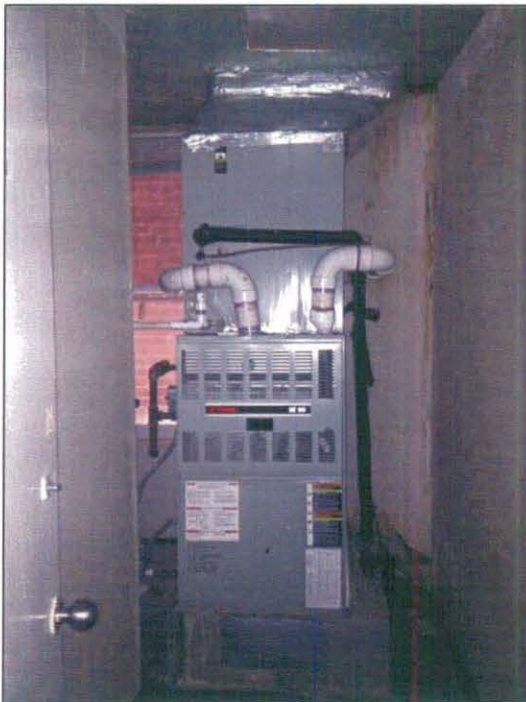
COMMERCIAL HVAC SYSTEM
