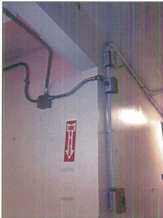
EXPOSED COMMERCIAL FIRE SAFETY EQUIPMENT
