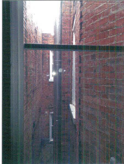
EXISTING NONCONFORMING COURT
