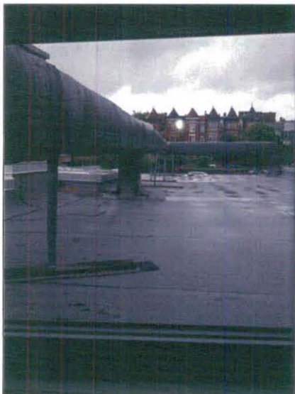
COMMERCIAL HVAC SYS.
