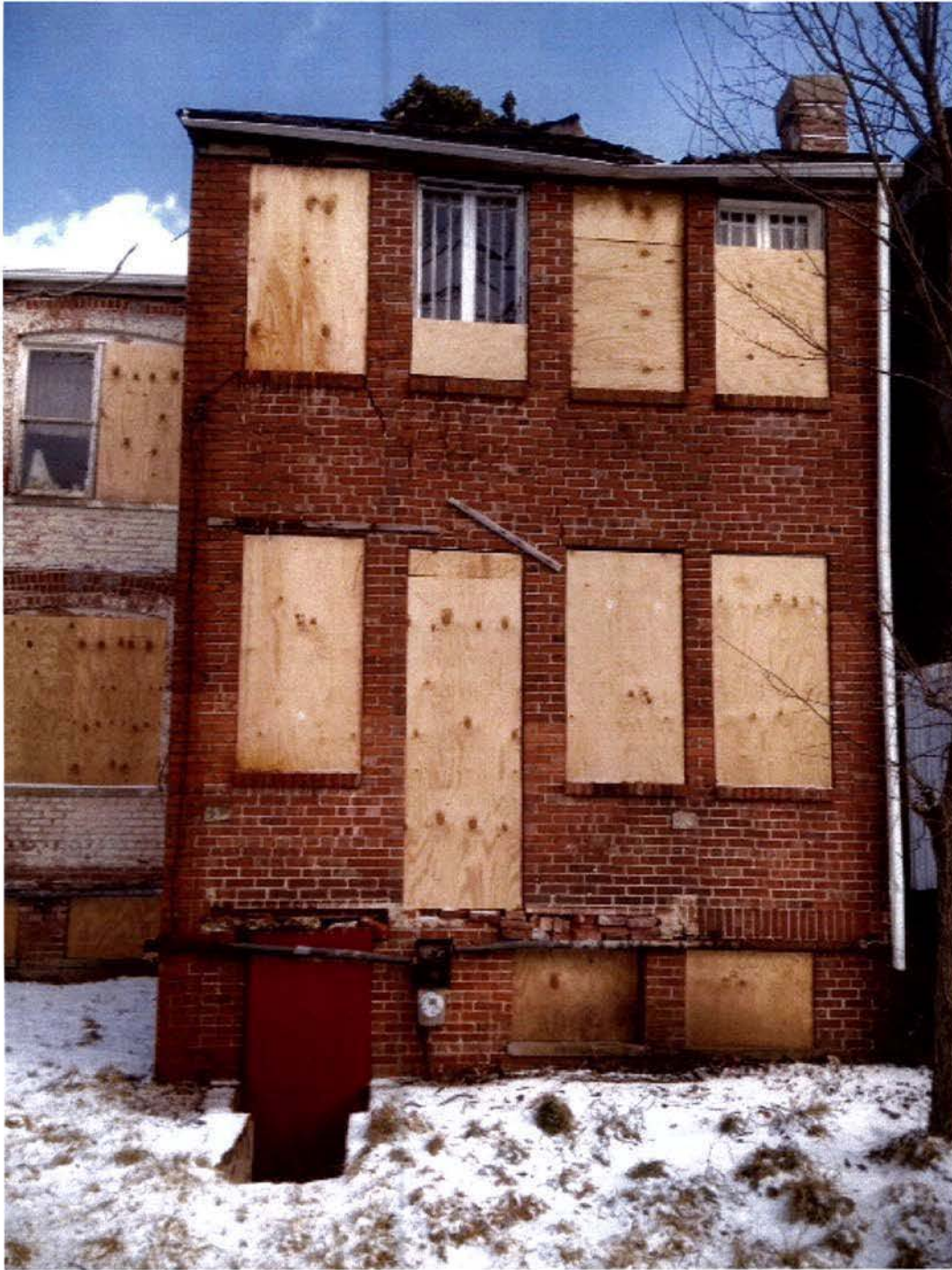
Rear Exterior- Masonry Structural Damage
