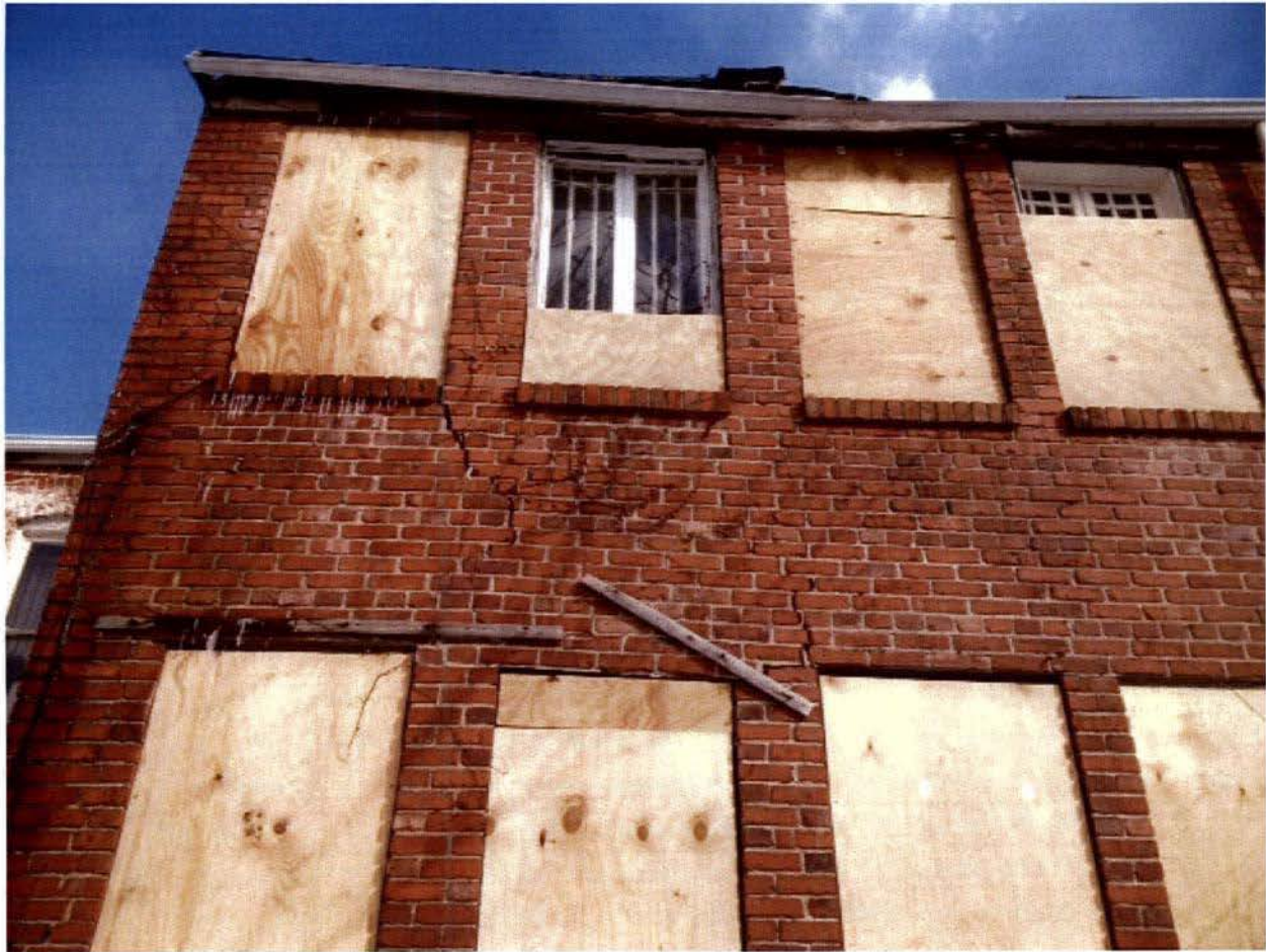
Rear Exterior- Masonry Structural Damage
