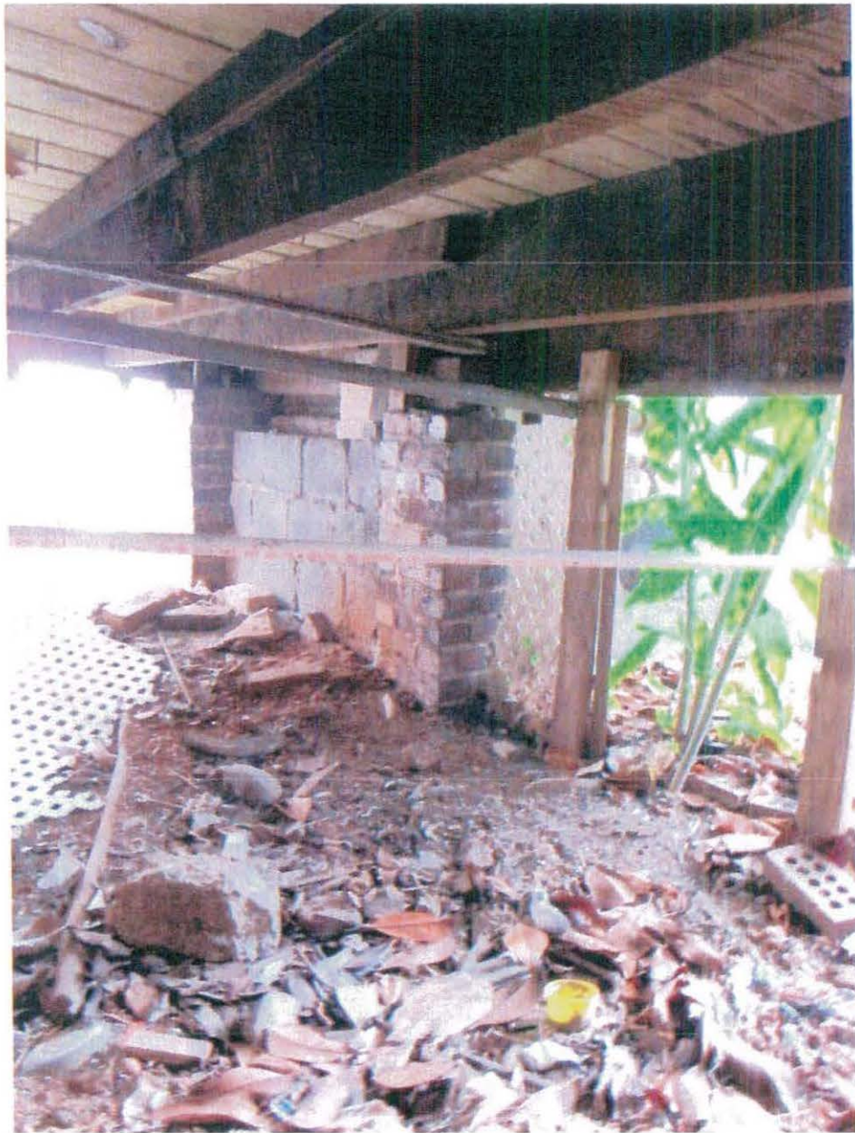
3614 Porch Pier Settlement
