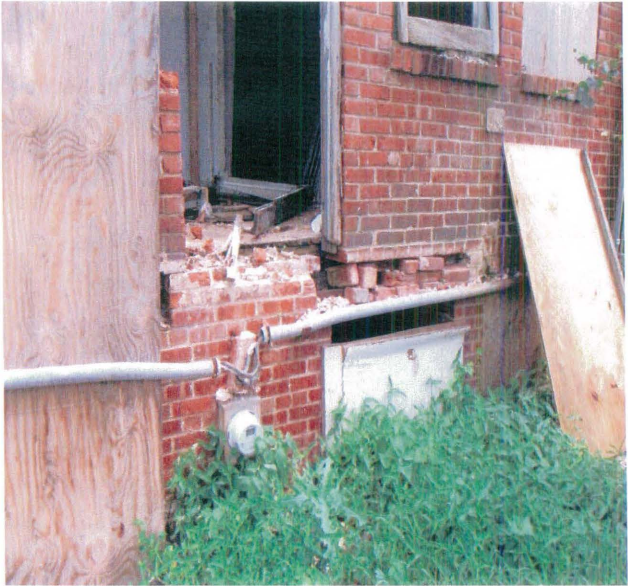
Settlement Damage to Masonry
