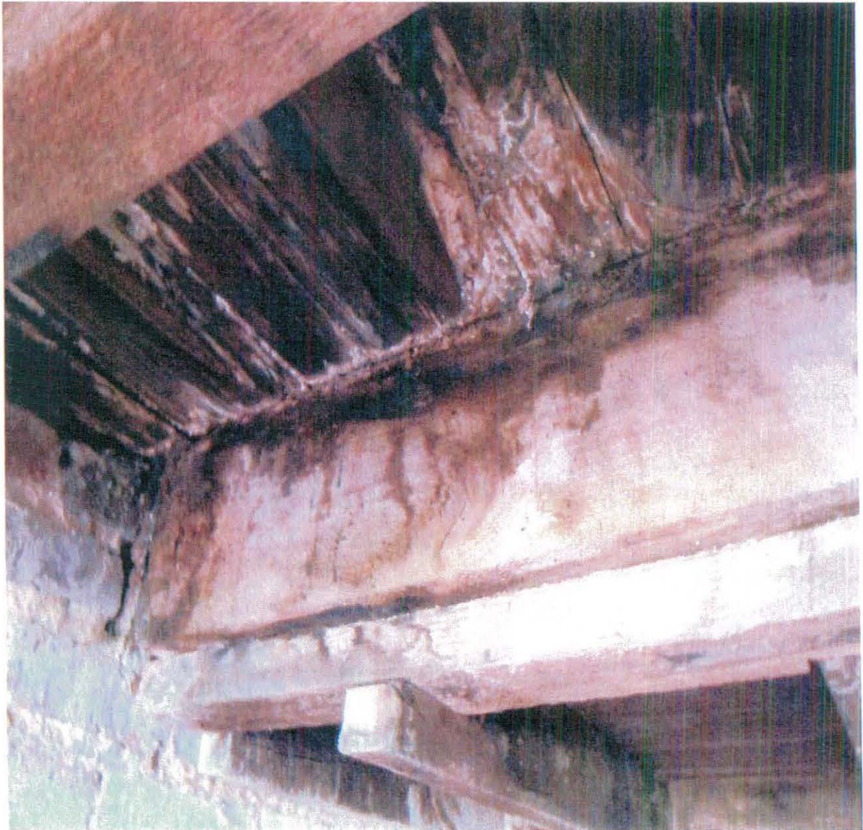
3612 – Mold and Termite Damage
