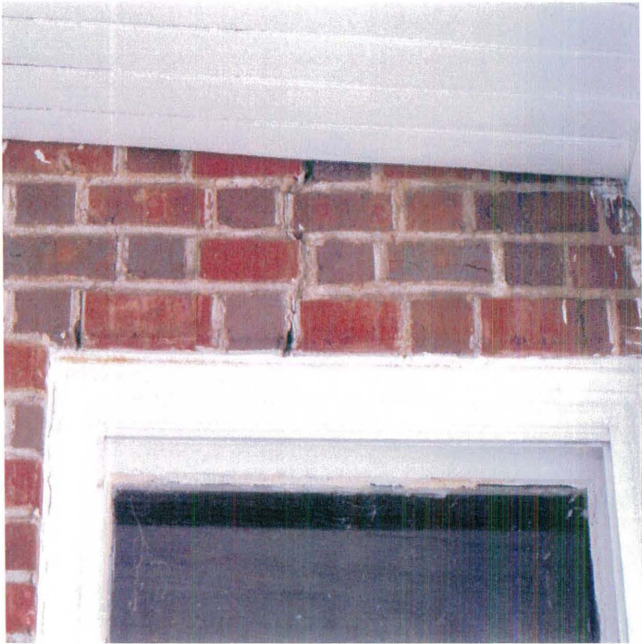
Settlement Cracks in Masonry
