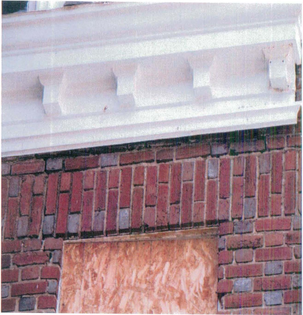
3614 Park – Mortar Deterioration and Cornice Spreading
