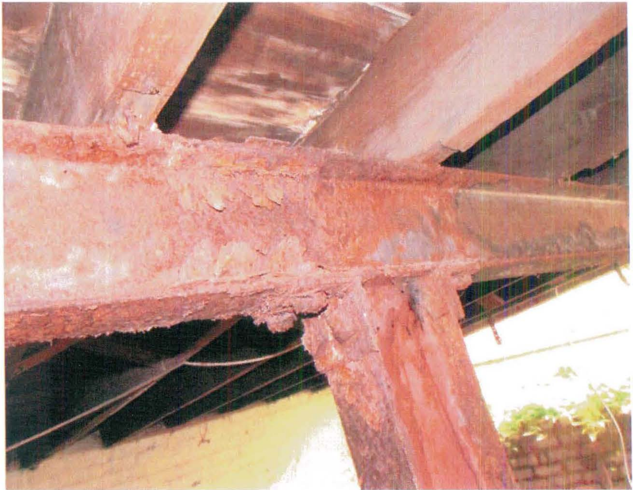
3612 Park – Rusted Beam and Column
