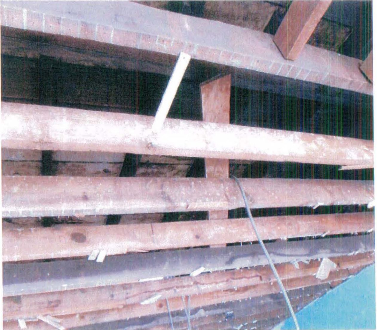
3612 - Mold on Joists
