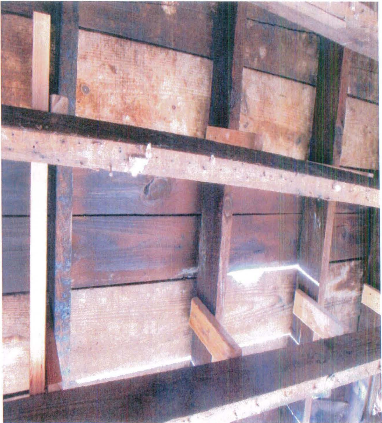
3614 Park – Hole in Roof and Mold Damage
