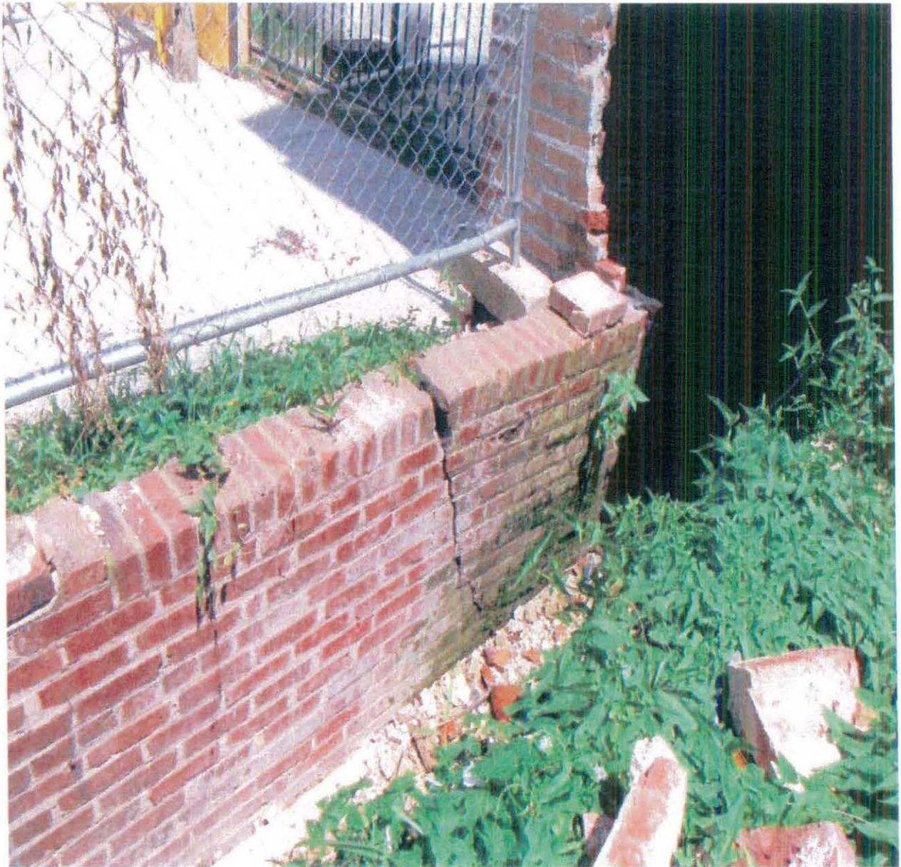
Soil Pressure and Areaway Damage
