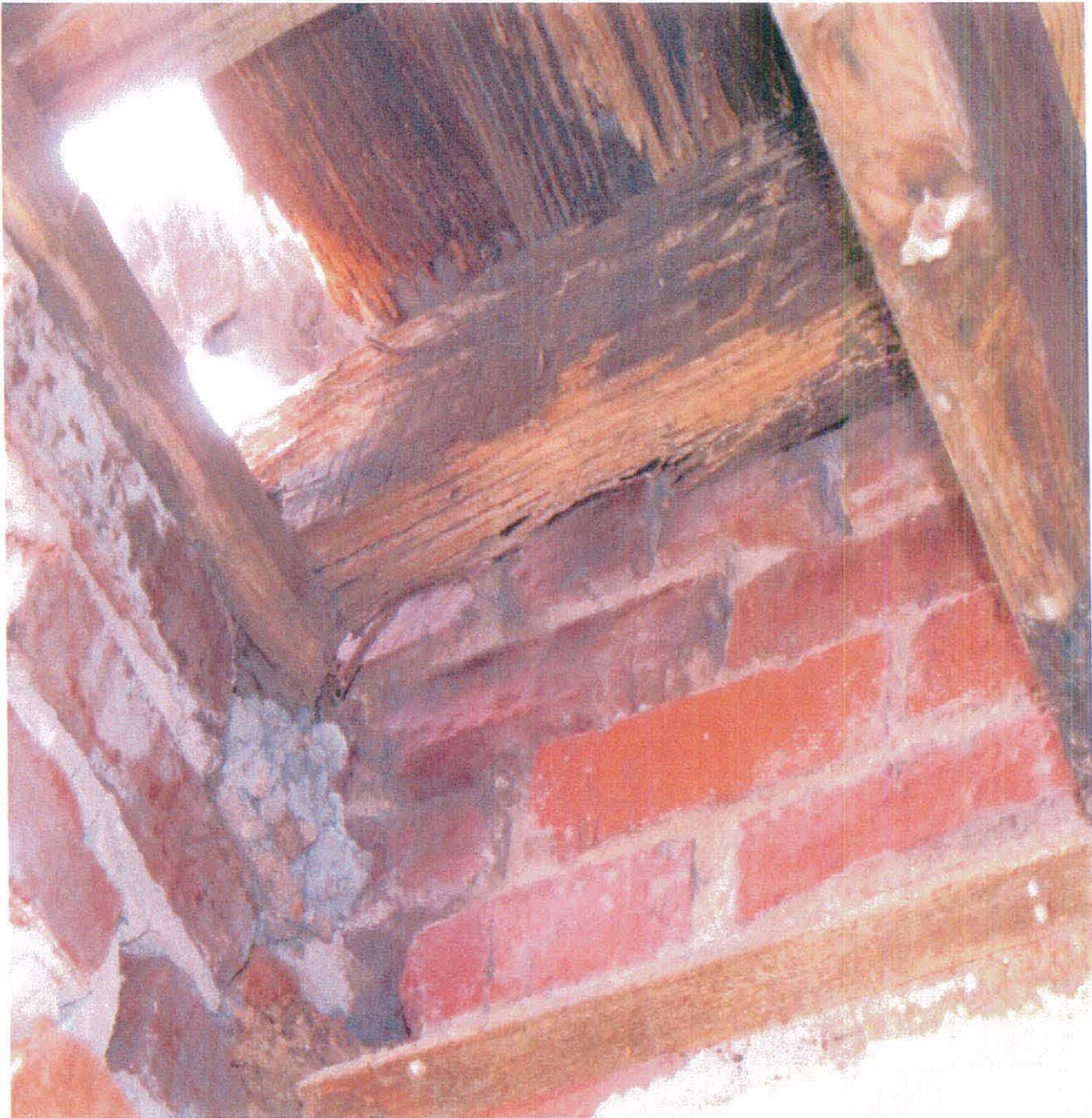
3614 Park- Termite Damage
