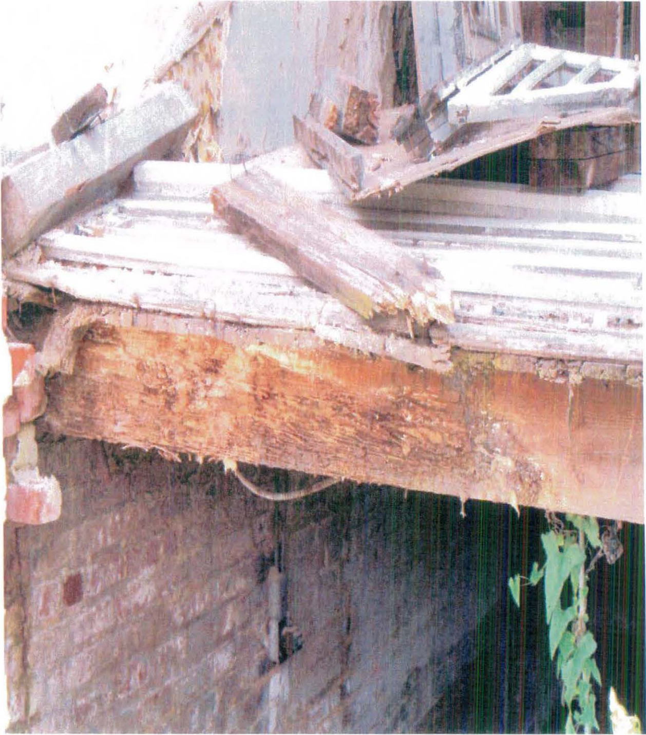
3614 Park – Termite Damage
