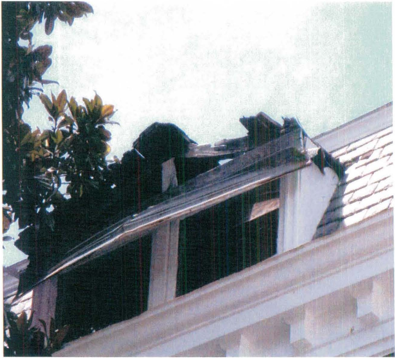
3612 - Dormer Roof and Window Damage
