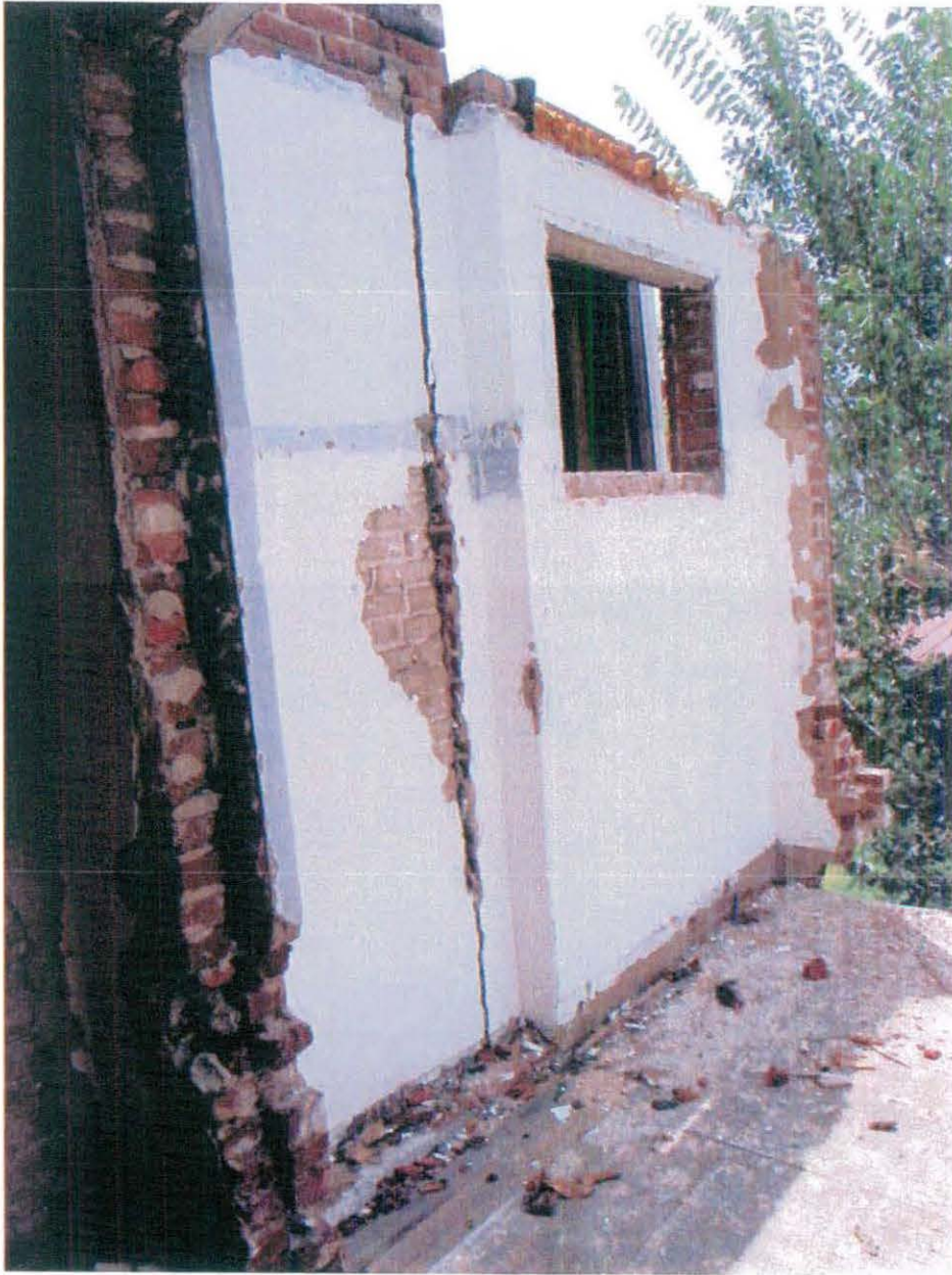
Unstable Brick Addition Had to Be Demolished
