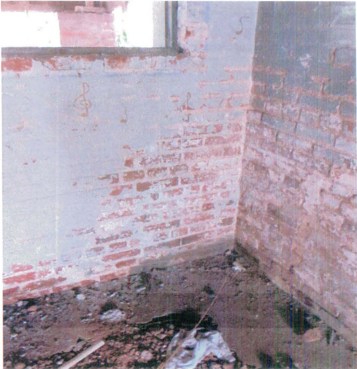
3612 - Slab Displacement – Mortar Deterioration
