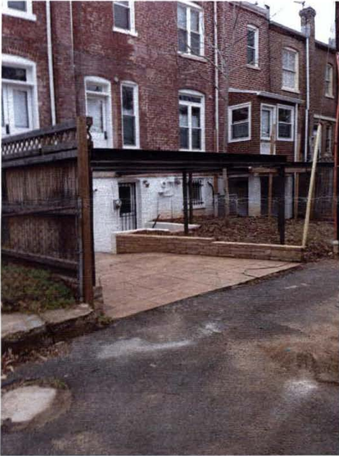
Photo #3: Work started in violation of zoning months ago
