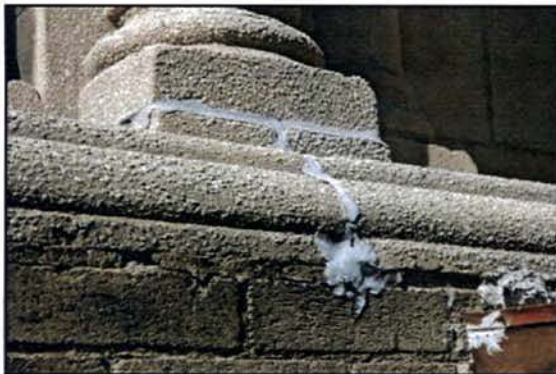
Left: Deteriorated brick mortar joints beneath open stone joints, improperly sealed with caulk.
