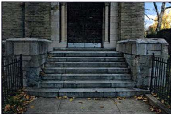
Top Left: Large areas of failed patch work and deteriorated stone on the South entrance knee walls. Bottom Left: South entrance knee walls and steps are heavily damaged. Right: Exploding cast stone on top of the right hand brick knee wall at the West entrance steps.
