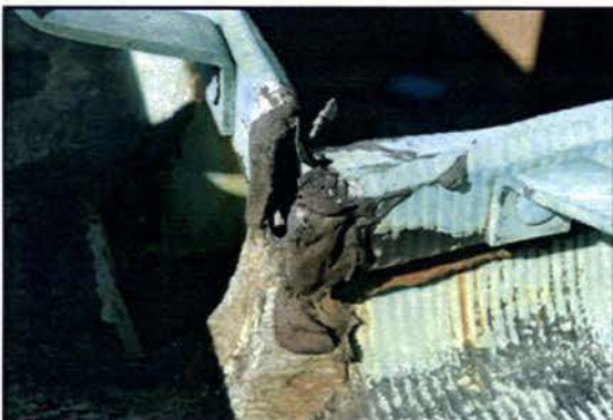
Right: Areas of flashing on the East sanctuary wall have little to no sealant.
