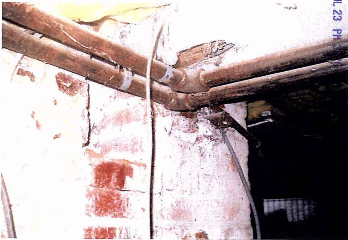
Basement- View of Hole for Missing Beam
