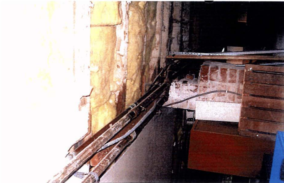
Basement Photo Showing a Slot for the Missing Beam
