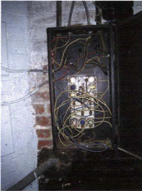
Fig. 3. Existing electrical panel.
